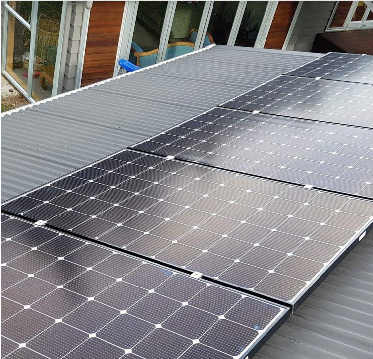
The Griffith's 4.8kW Solar Power System "Thrilled to date with the system"
