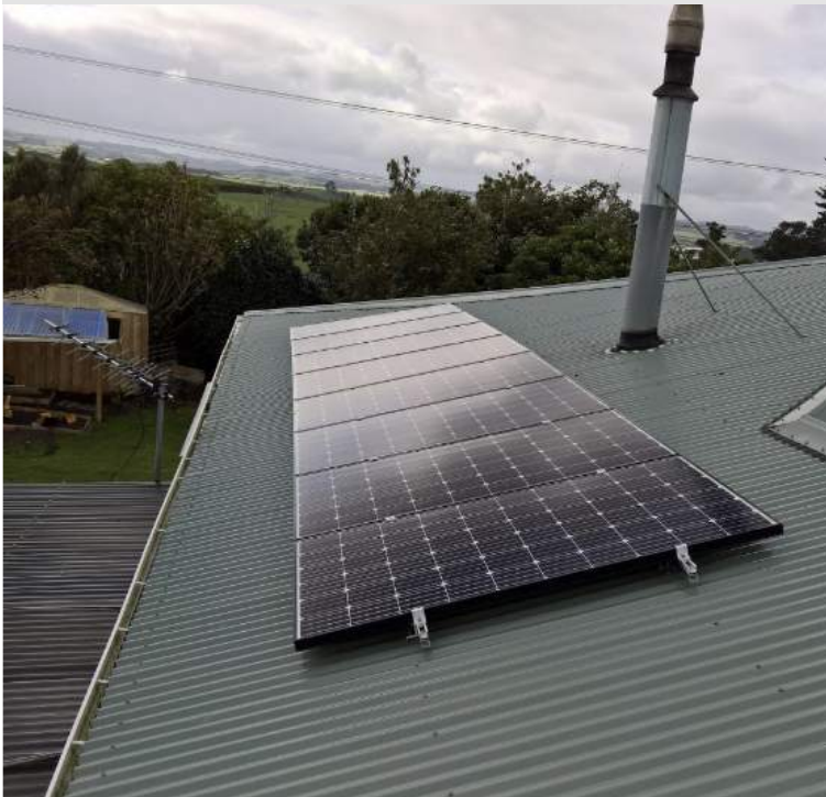
The Wright's 2.4kW Solar Power System "It's nice to see more people going solar"
